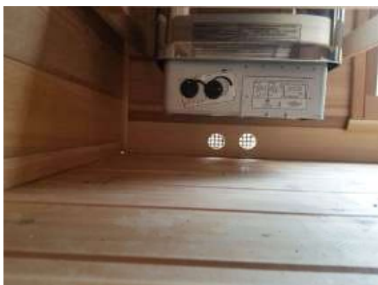
Inlet under electric heater on Back wall
